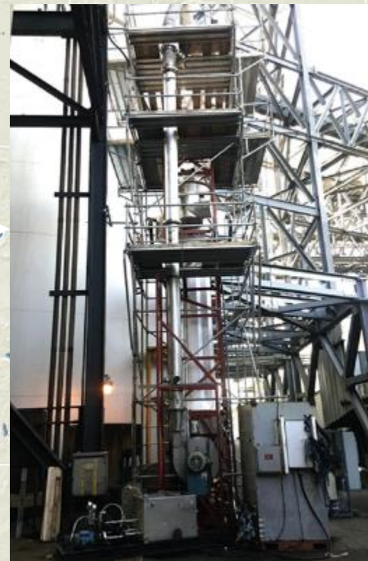
Wet ESP Installed at MRY
